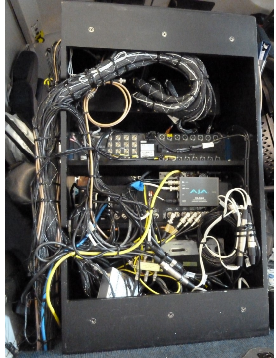
Rear of Photographer's Control Panel
