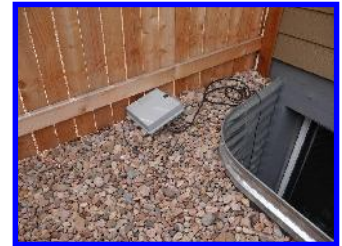
SG-237 Embedded in Weather Resistant Enclosure - No Snow!
