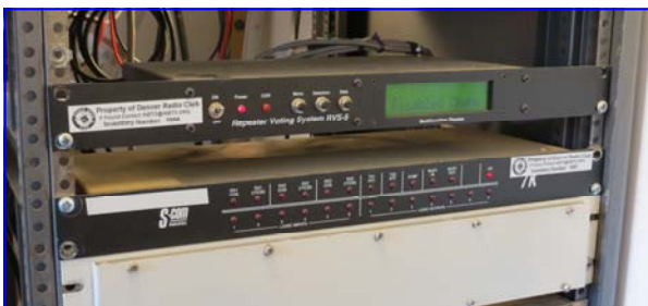
The Voter Panel (top) and the Repeater Controller (bottom).
